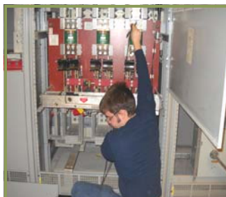
Testing of ground fault switches
