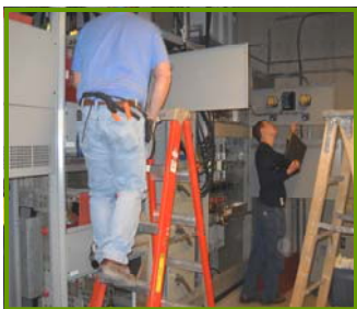
Opening main switch gear
